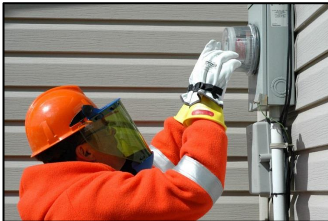
2Meter Technician removing meter from residence.
